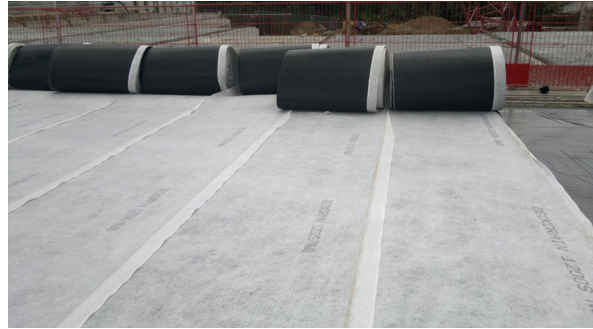
Fig 8: Deckdrain is butt-jointed and the geotextile overlap prevents soil ingress at the seams
