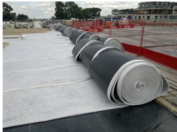
Fig 2: Rolls of Deckdrain are quickly laid directly onto waterproofing on concrete roof slabs
