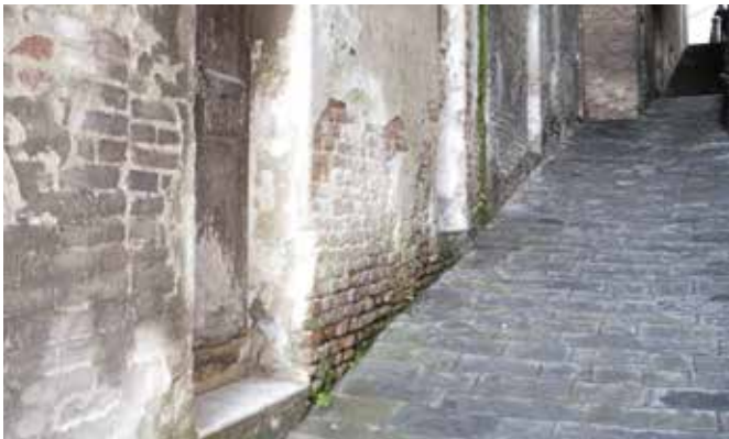
Destruction of render and mortar joints
