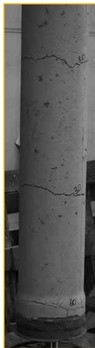
second crack (300 N/mm 2 )
